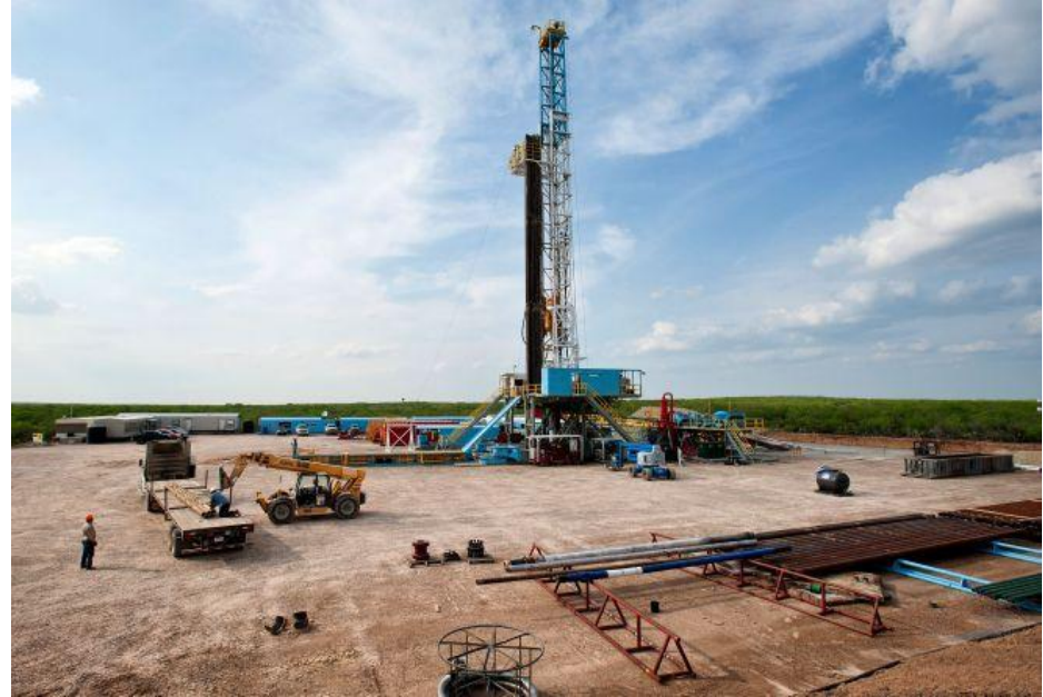
Fig. The Orion Drilling Co.'s Perseus drilling rig stands near Encinal in Webb County, TX
